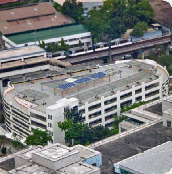
Providing all the energy needed by the parking building, solar panels at the top of the multistory car park of ADB Headquarters in Manila, Philippines, demonstrate the distributed generation potential of solar PV in urban settings.
