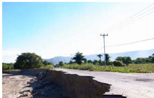
Timor-Leste road destroyed by flooding
