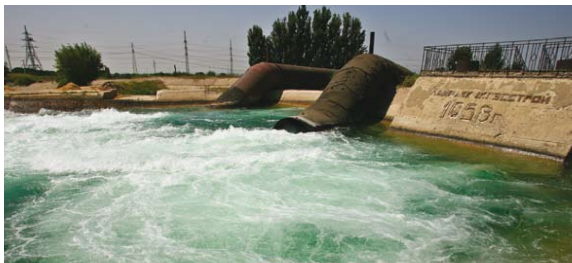
A refurbished reservoir in Khojabakirgan is part of the Agriculture Rehabilitation Project.
