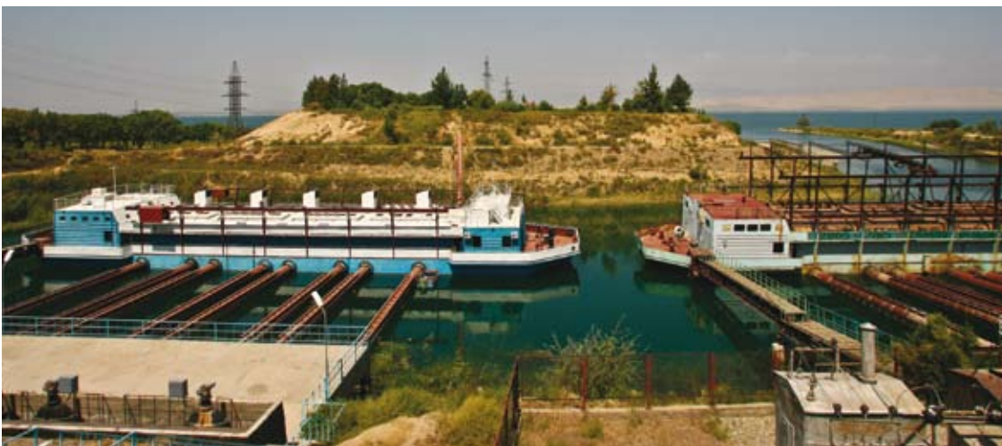
This floating pump station is in Khojabakirgan, Bobojon Gafurov District, on the banks of Kairakum Reservoir.
