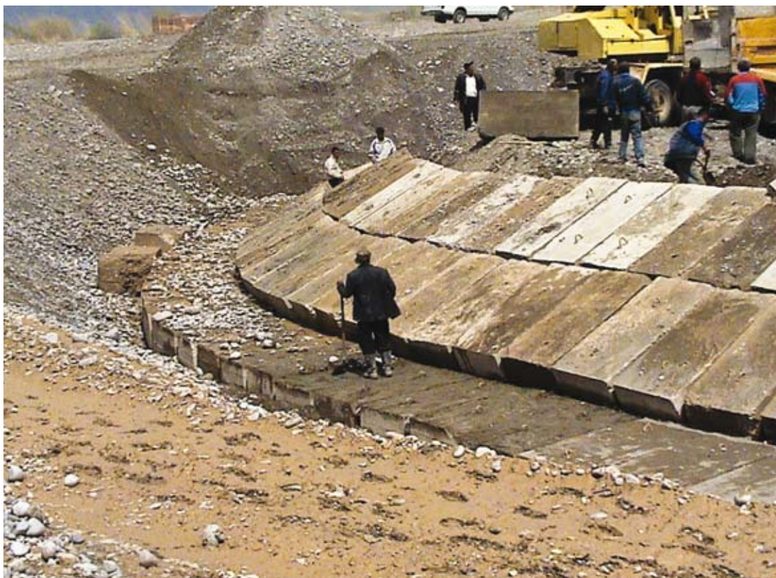
ADB is funding a flood risk management system in Khatlon Province.
