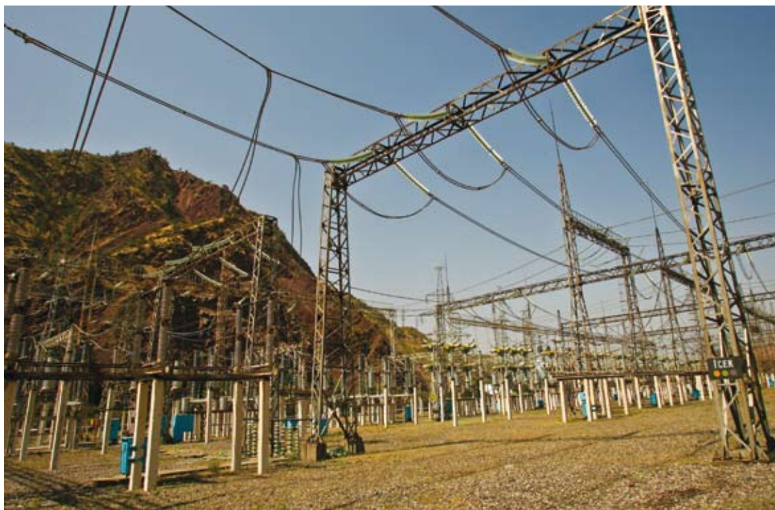
This 220 kV switchyard and a nearby 500 kV installation at the Nurek hydro power plant will be replaced with modern gas-insulated switchgear through the ADB Switchyard Reconstruction Project.
